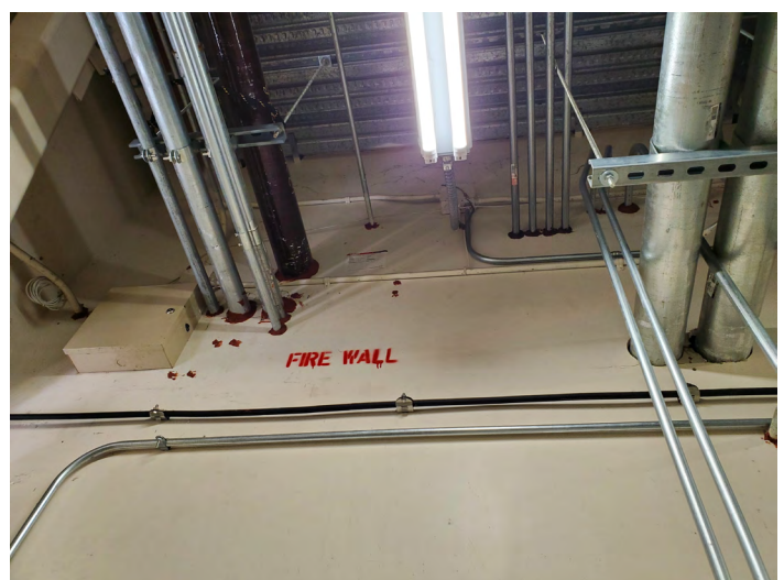
Interior fire barrier with fire stopping.
