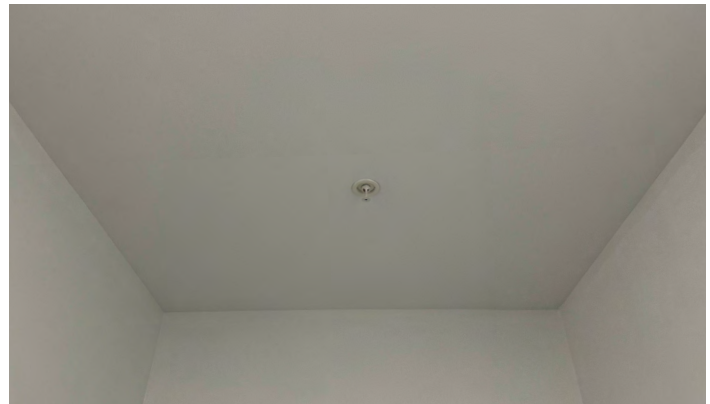
Finished drywall ceiling, which limits the passage of smoke. Fire and smoke partitions can terminate at a drywall ceiling.
