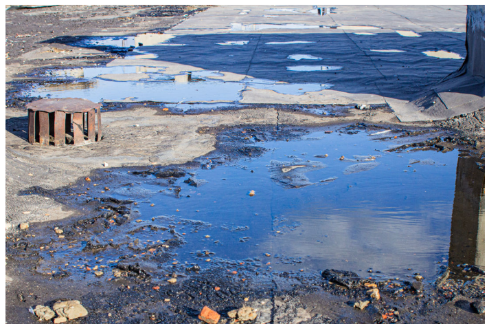
New MSBC requirements help identify roof bays that are susceptible to becoming unstable from ponding rainwater.
