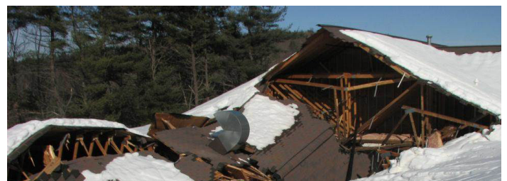
Many new snow load requirements provide guidance on items that were previously left to the engineer's judgment.
