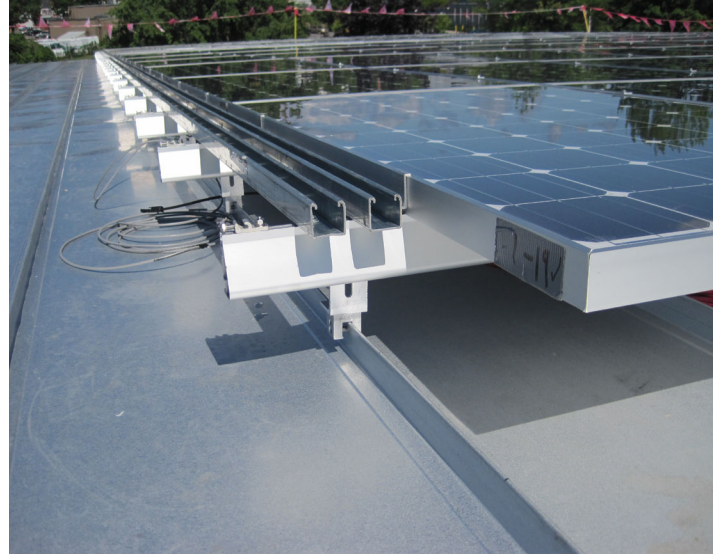
The new MSBC provides substantial guidance on wind uplift pressures on roof-mounted solar panels.
