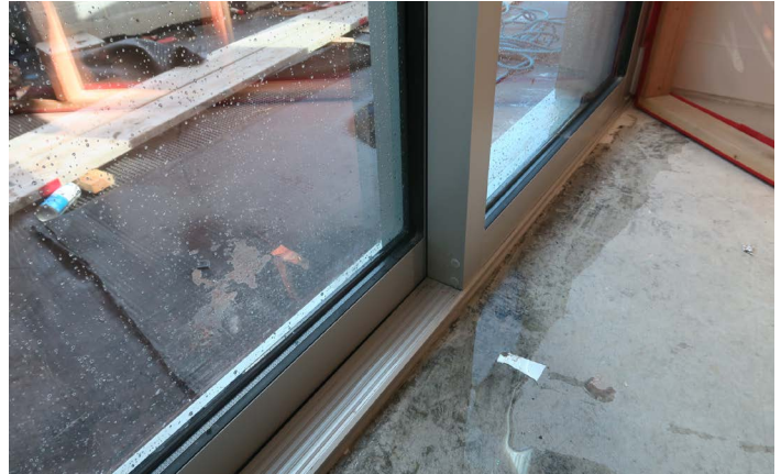
Leakage from sliding door sills
