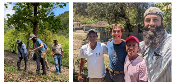
In May 2022, Keith Nelson traveled to Ocotal, Honduras, to help lay out and begin construction for 3.5 miles of water transmission line. The project includes ongoing design, monitoring, and reporting from the U.S., and its next phases are a storage tank and transmission network.
